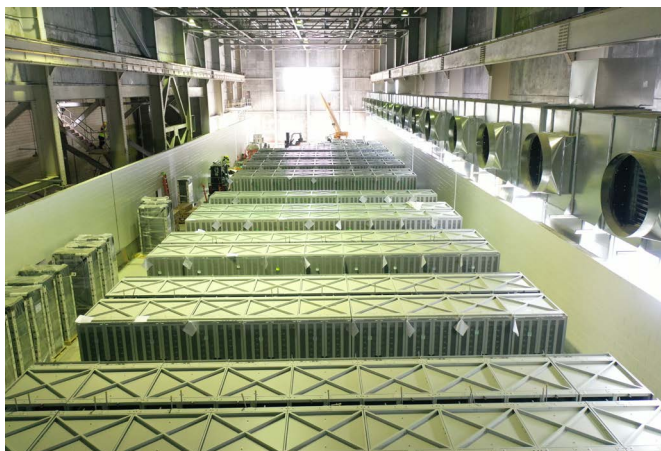
Supplying 1.2 GWh-scale power grid ESS to Vistra in the U.S.
